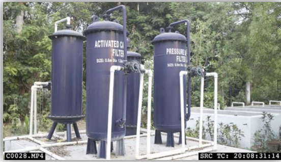
Waste Water Plant
